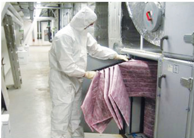
Figure 9: Personal protection equipment for filter replacement
